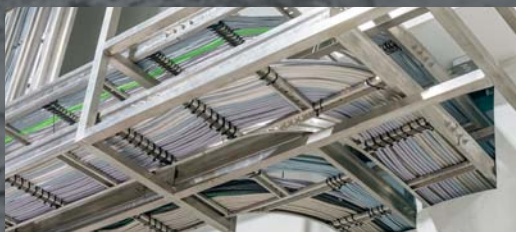
CABLE TRAYS AND MECHANICAL INSTALLATIONS ON UNCRACKED CONCRETE
